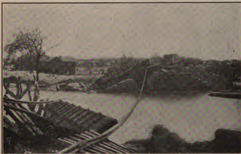
FIG. 4.—The Sullivant Ave. Subway, on the B. & O. R. R., Columbus, Ohio, after the March, 1913, flood.
